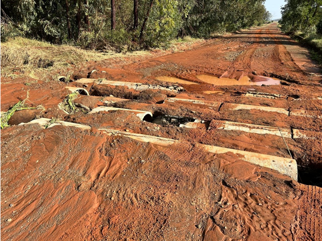
Figure 6. Culverts on S426 completely exposed after a rain storm because of being blocked & graded open by a lack of a gravel layer – photo supplied by Willie Hertzog, Geluksdam Farmers Association – 12-02-2025
